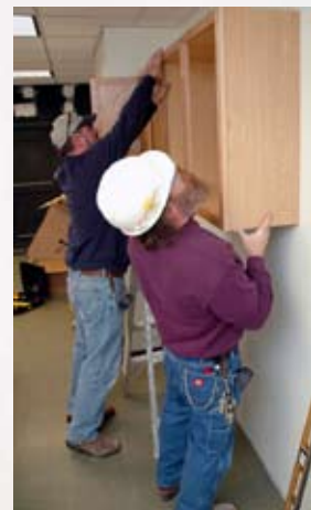
A renovation crew from Penn State's Office of Physical Plant installs new kitchen cabinets in the new student commons room.
